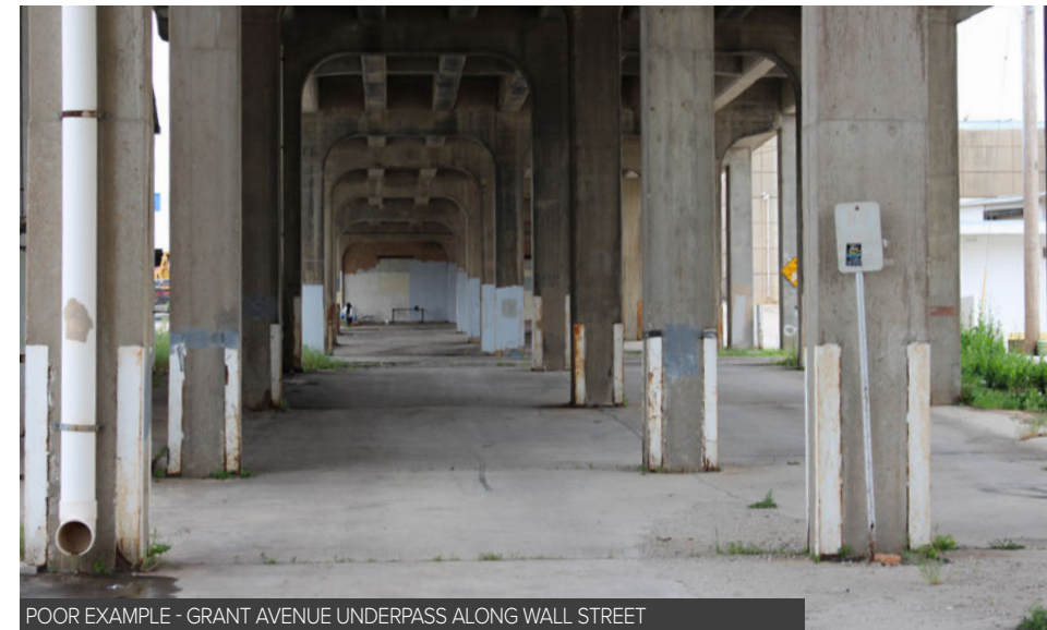
POOR EXAMPLE - GRANT AVENUE UNDERPASS ALONG WALL STREET
