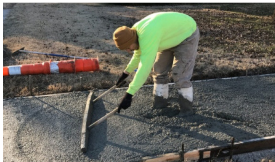
Caption: Approximately 3,714 linear feet of new sidewalk were constructed in February 2020 in the Delaware neighborhood, thanks to the City's Neighborhood Works capital improvement grant program.
